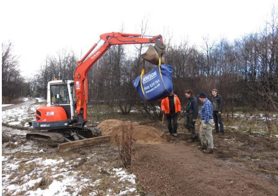
Figure 2: The bee bank being created with the help of volunteers from TCV and a contractor on the 12 th of February 2018.
